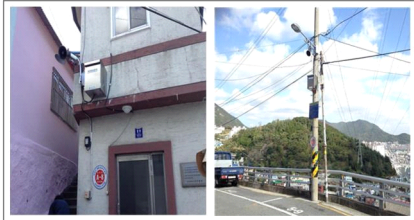
Figure 10: Special Lighting Installation
